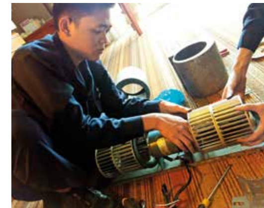
Thu Ya Win, a graduate from the SMVTI course "Residential Air-conditioning" during his internship at the Fairmont Hotel in Singapore.
